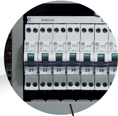
MCB's for line protection
